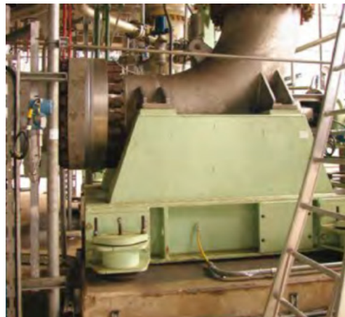
The axial flow circulator pumps for loop reactor
