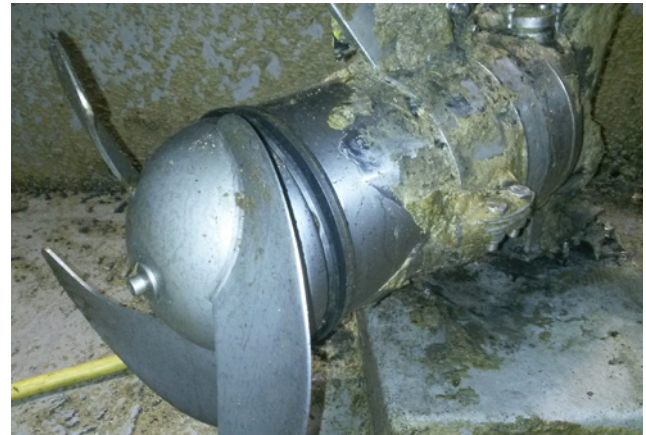
Mixer inspection after six months of operation
